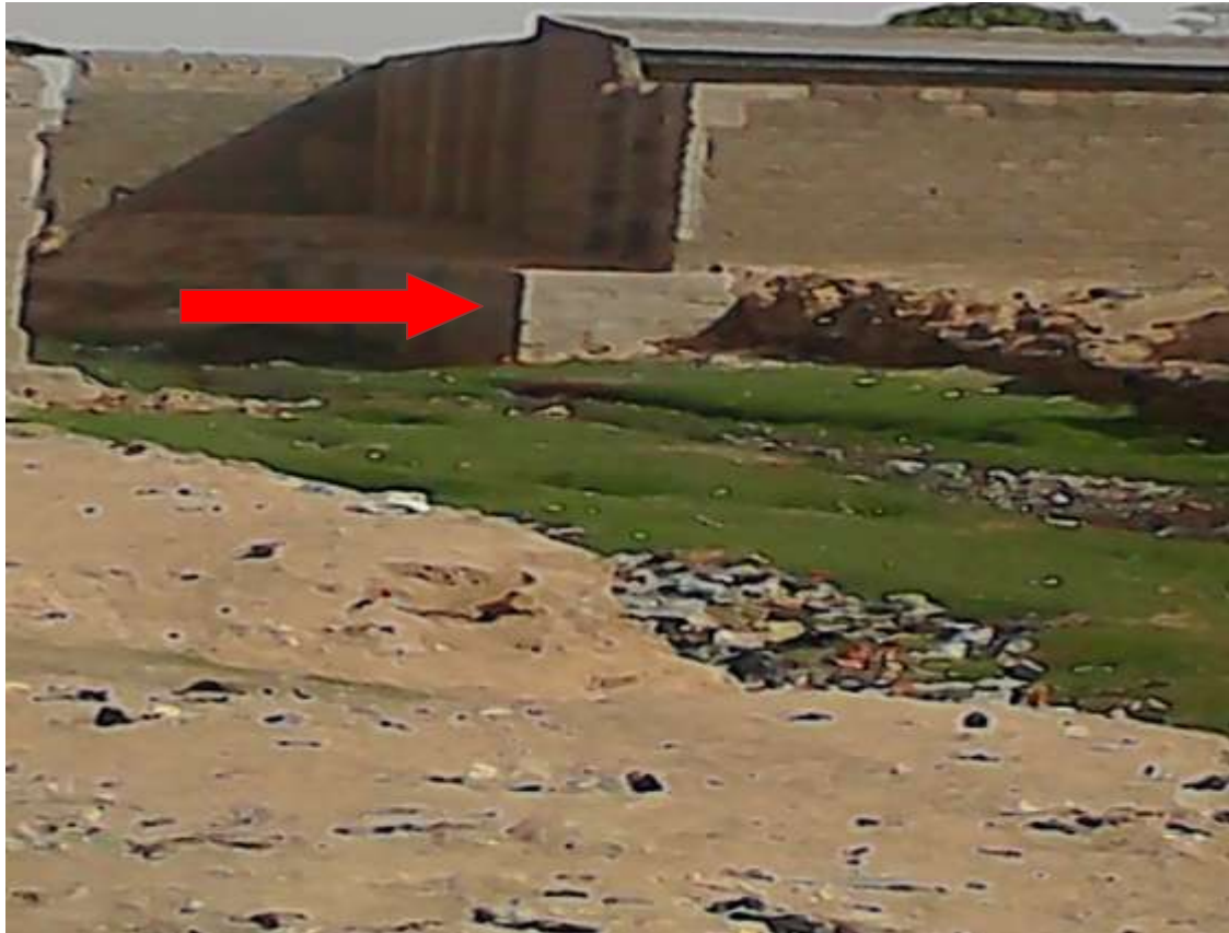
Plate 1: Construction of retaining wall/raising house up above flood level as a coping strategy to flood (Picture Location: behind Alliance bread, Kofar Kaura, Katsina).
